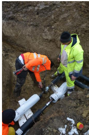
Assembly expansion bend
