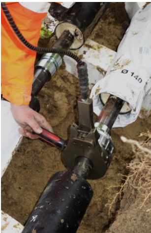
No room for welding
