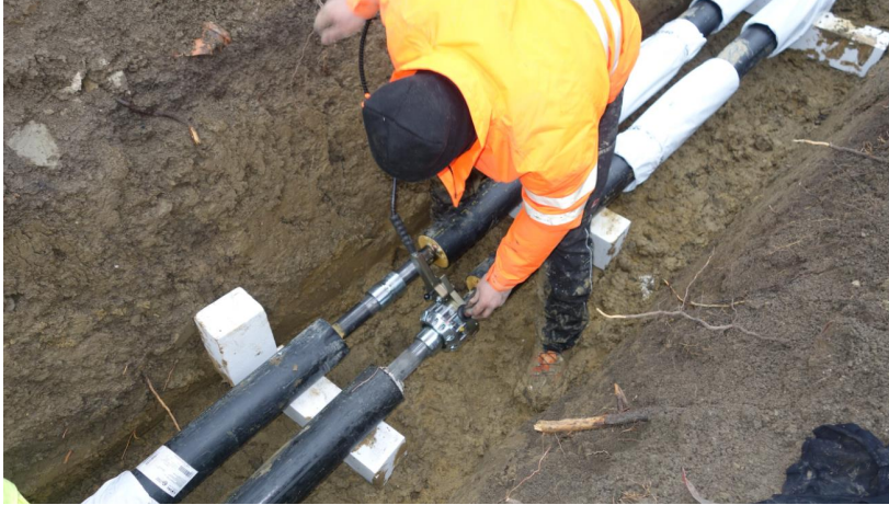
Pressing (approximately 80 seconds per installation) – one battery charge was sufficient for the whole project.
