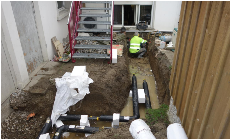
Condition at house entrance: Does not allow for welding.
